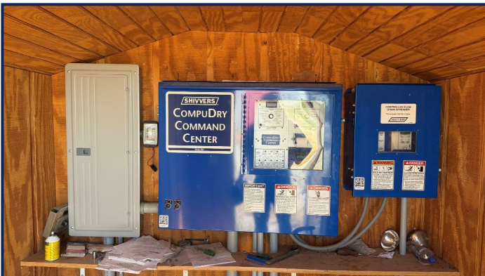
Grain Dryer Controller
