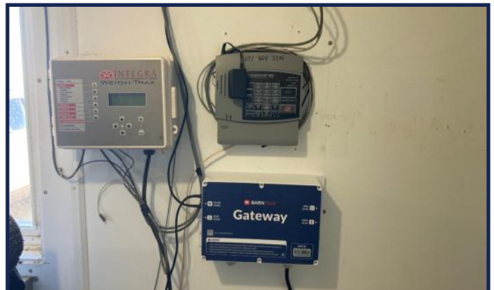
Barn Talk Alarm System
