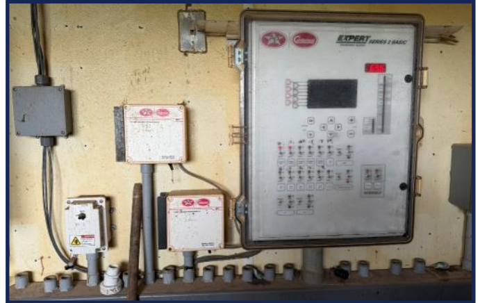
Gestation Room Controller
