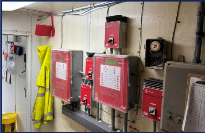
Gestation Room Controller
