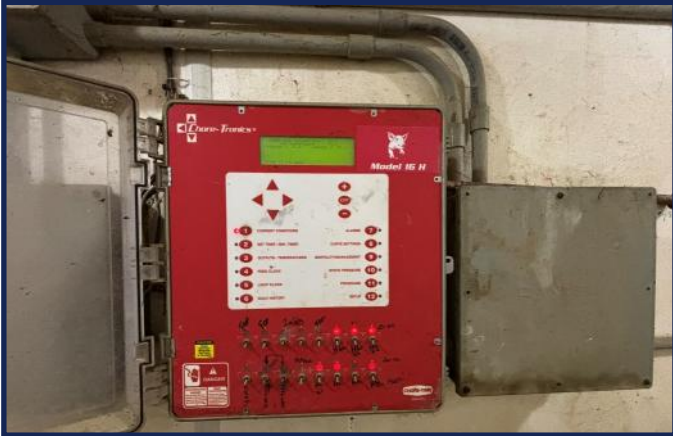
Farrow Room Controller
