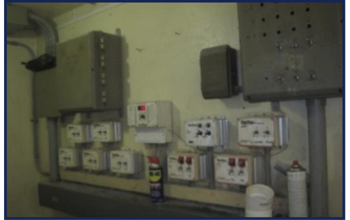
Gestation Room Controller
