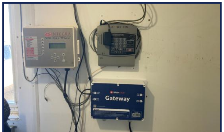
Barn Talk Alarm System
