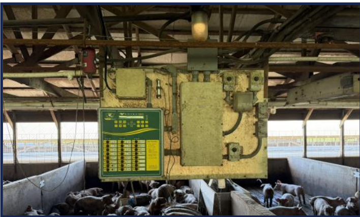
Controller /Backup Thermostats
