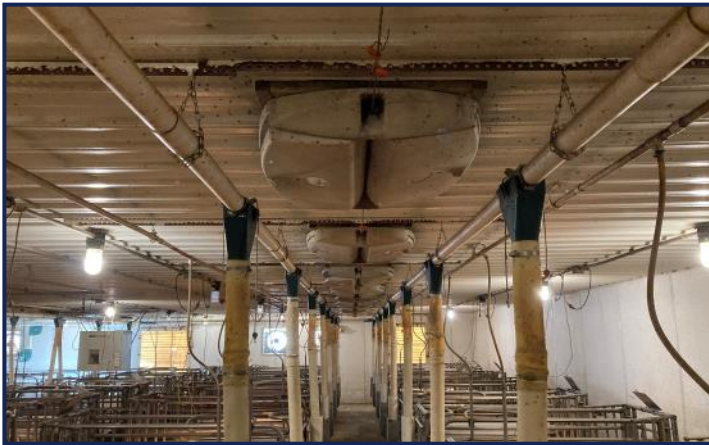
Room Air Inlets
