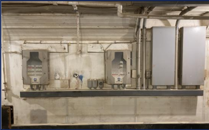
Gestation Room Controller
